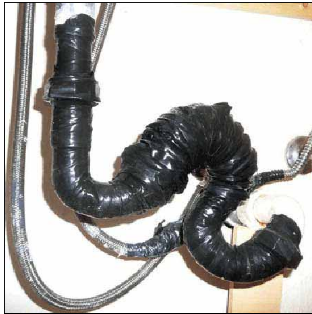
Leaky drain - out of duct tape, then use electrical tape
